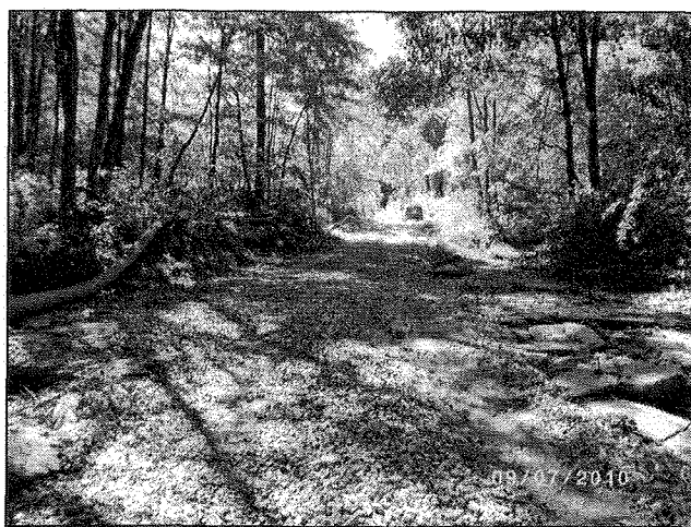
Blake Fork after having stone and gravel spread in the stream to create a roadway
