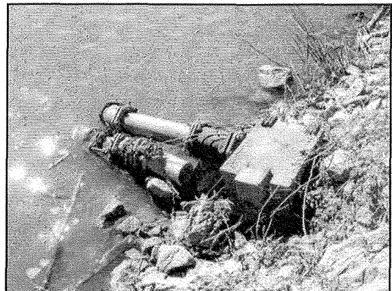
This is the second underwater extension of Arkla's river outfall. The blue piping was added in September 2007, shortly before the welded bypass was added at the facility. The piping was added to hide the illegal river discharges.
