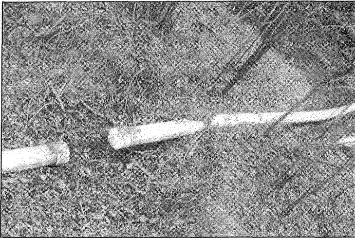
Piping that was removed from Arkla's river outfall pipeline. This was the only place where the otherwise underground pipeline was exposed. The section of piping was removed by a contractor at John Tuma's request as part of a cover story created by Tuma claiming that the facility was incapable to discharge to the river because the line was capped.
