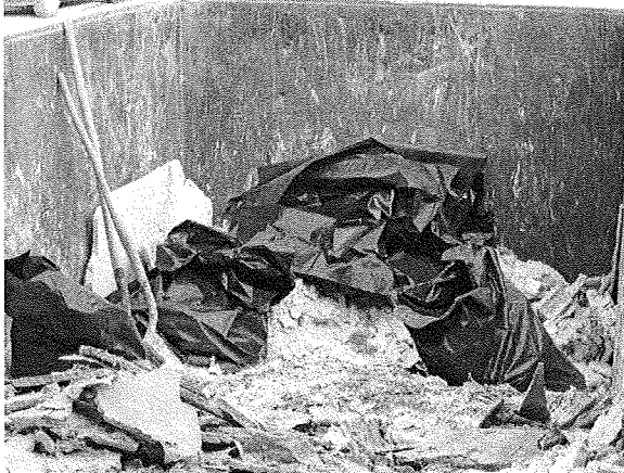
Dumpster containing friable asbestos. NYS-DOL inspector observed two unprotected workers inside this dumpster, including a 16 year old.
