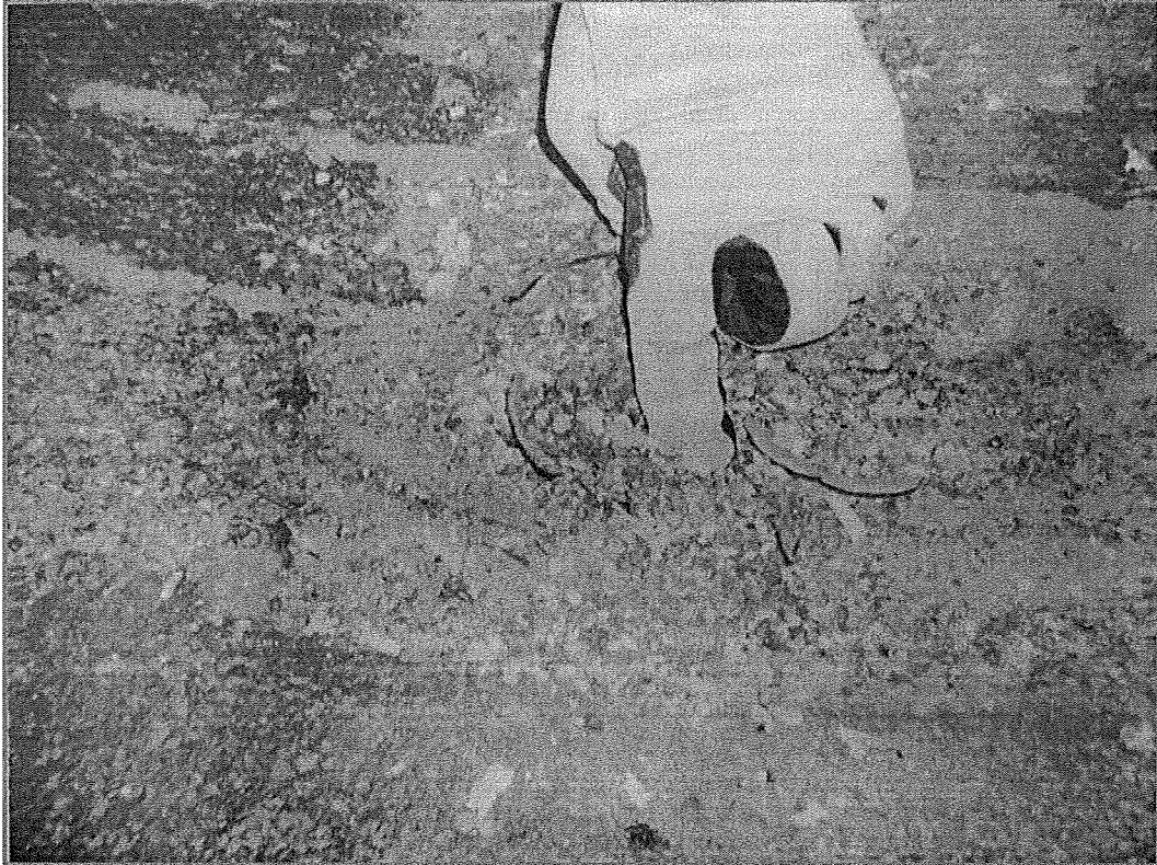
UST 87 Octane internal view: gel deterioration
