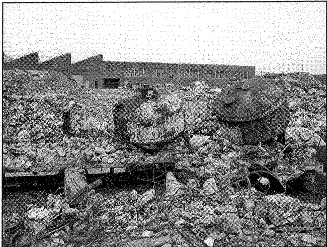
Debris piles with stripped tanks
