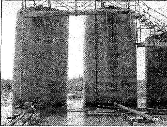
Oil pooled around T & F storage tanks
